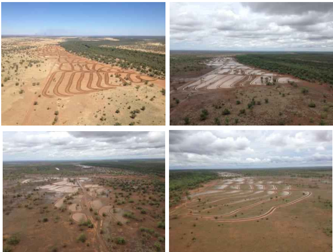
Figure 15. 'Go Go' Station rehabilitation pond banks: Top L. At bank establishment; Top R. First filling with water in the first wet season; and Bottom L. and R. Ponds with water during the first wet season (Photos: Rick Ford).
